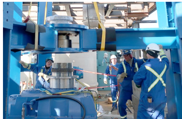
Installation of equipment to expand a carbon capture pilot project at Pikes Peak South.
