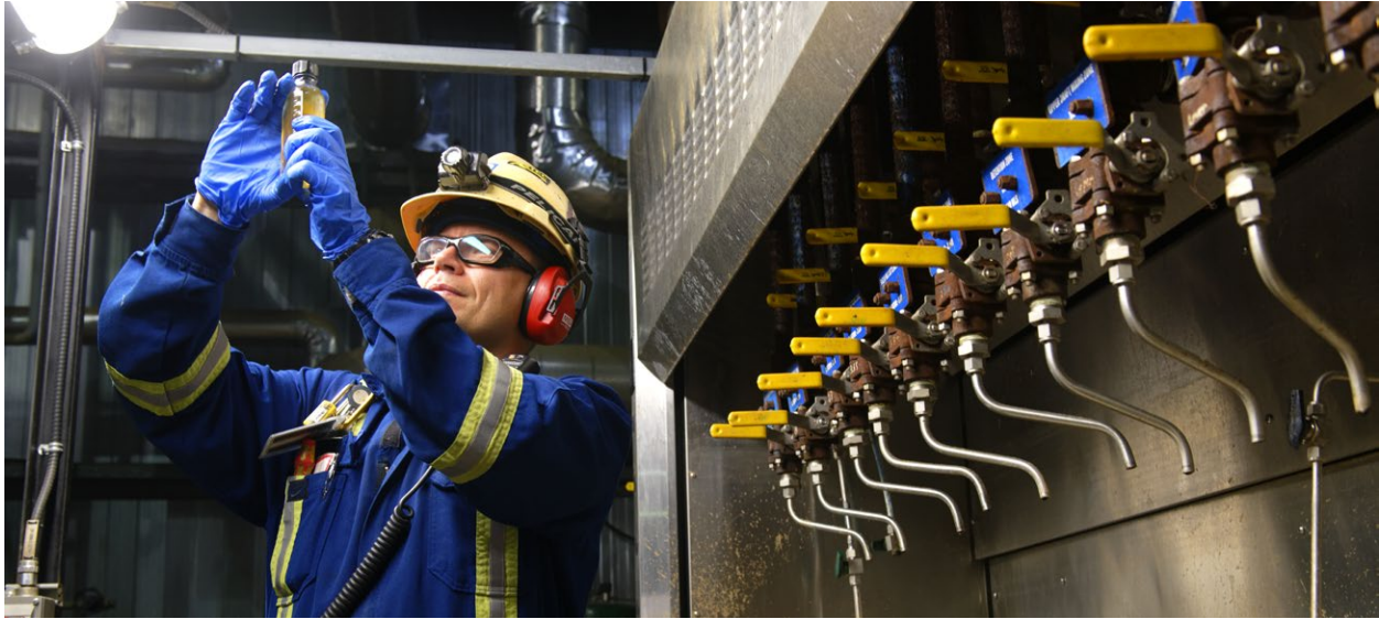
More than 82% of water used to generate steam at Tucker is recycled produced water.
