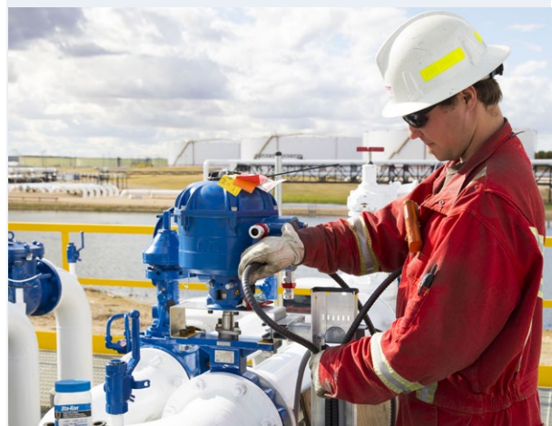
Pipeline integrity is a focus at our Hardisty Terminal.
